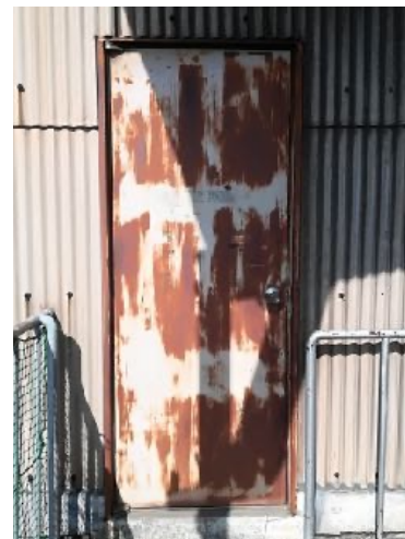
Hoist load-in entrance: 3F south; door size W730 × H2100 mm
